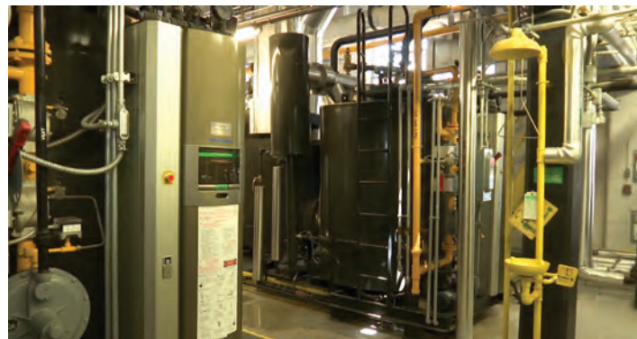
With the assistance of Boiler Masters Inc., Southeastern Health installed four EX-200 SGO Gas/Oil Series High Pressure Steam Boilers in their energy plant and a single 100HP unit in an off-site laundry facility.
