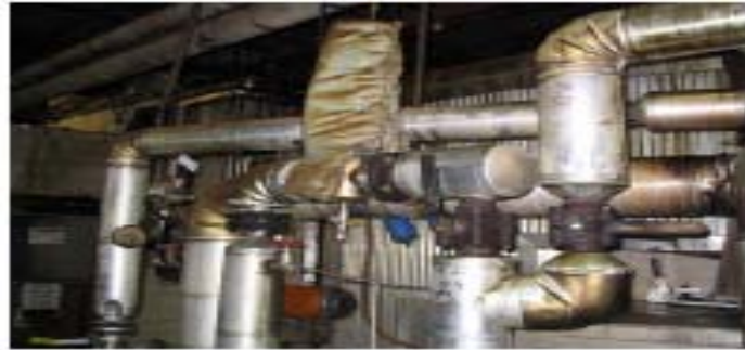
Non-Best Practice Piping to Agglomerator
