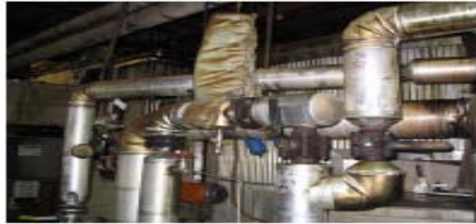
Non-Best Practice Piping to Agglomerator
